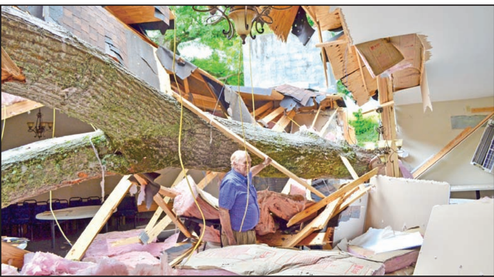
Another angle on the damage from the downed oak tree at Friendship Baptist Church. Photo by Lowell Nicholson
